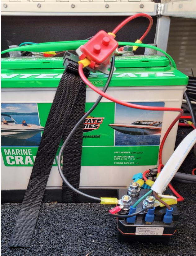
autobimini lite reversing contactor located near the battery
