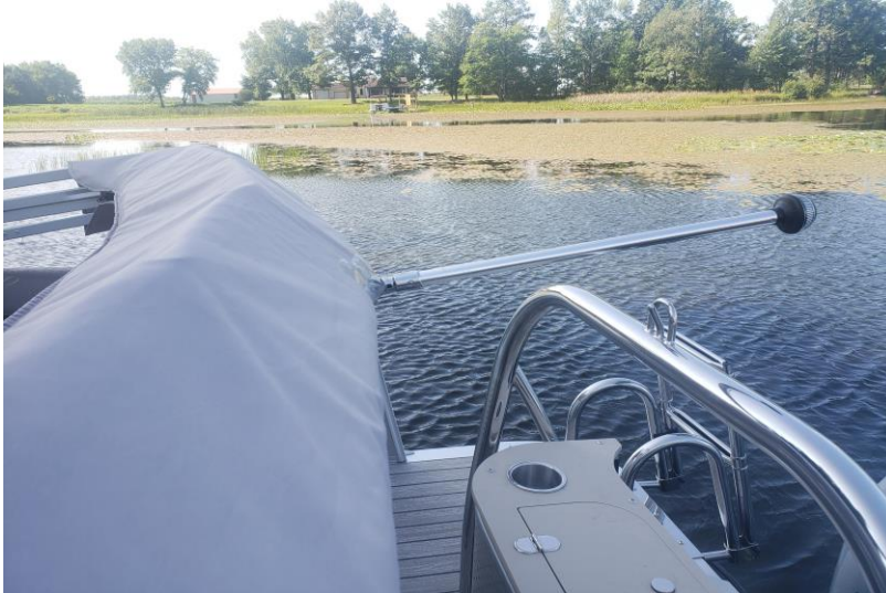
Navigation light installed on 4 th arch. Access holes are built into canvas and boot
